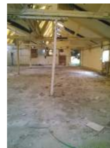
Structures verticales instables
